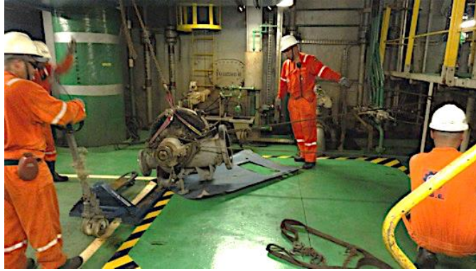
Figure 4 - Users assemble a system with hoists and cables to place the pump on the pallet truck
