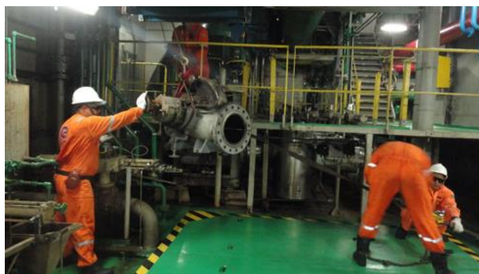
Figure 3 - Users pull the pump with the tirfor to get past the interference
